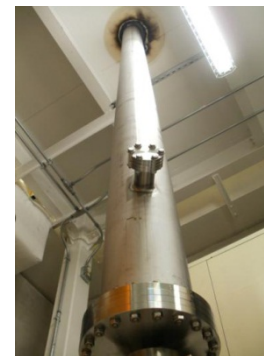
Cryogenic Container located at MSFC (below deck)
